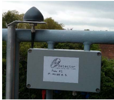
Automated DETECTOR Roadside Unit
